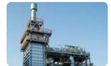
Waste liquid combustion furnace
