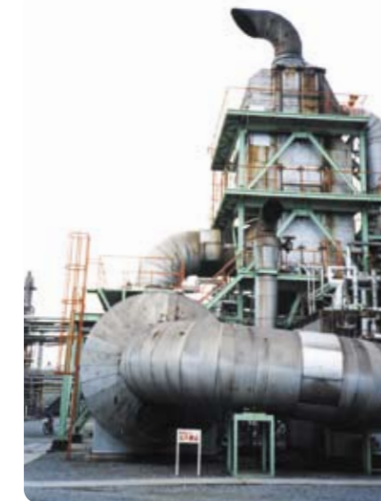
Flue gas treatment system
