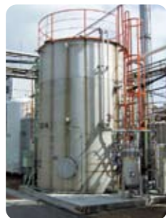
New tank for reclaimed water
