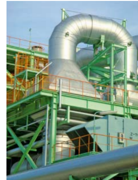
Flue gas treatment system
