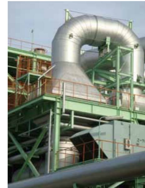
Flue gas treatment system
