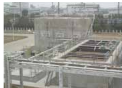
New activated sludge treatment facility
