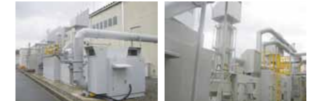
Exhaust gas treatment facilities
