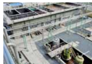
New activated sludge treatment facility
