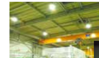
LED lighting (production building)
