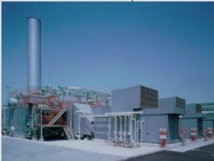
Cogeneration system in Himeji Plant
