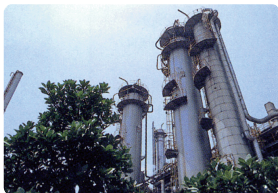
Ethylene oxide production equipment
